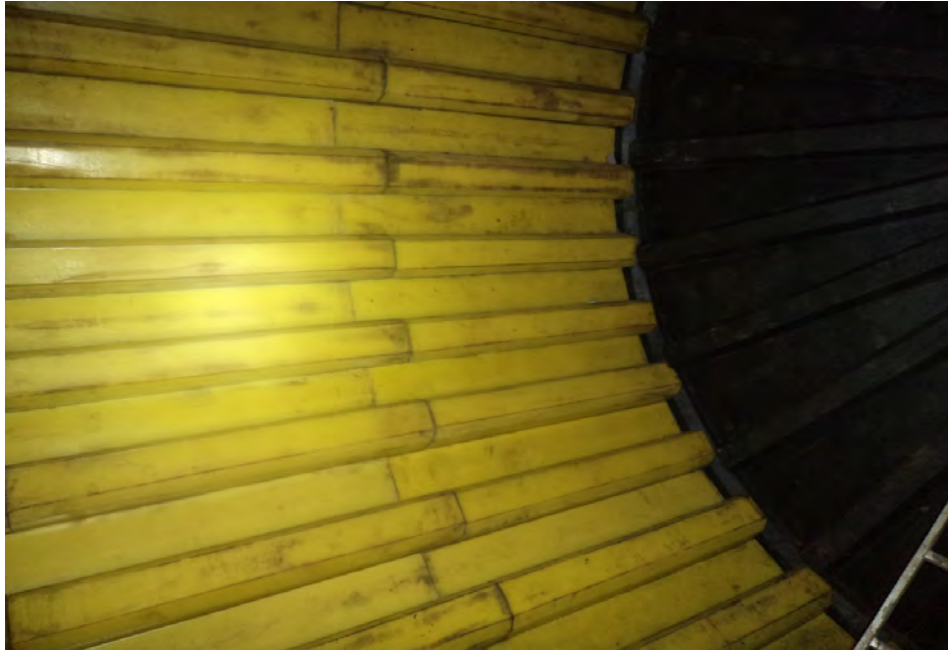
Ball mill LPUR lifter bars and liners
