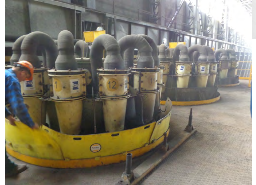
ZAM Kety hydrocyclones with PUR inserts Worker is fixing tailor made bath cover plates
